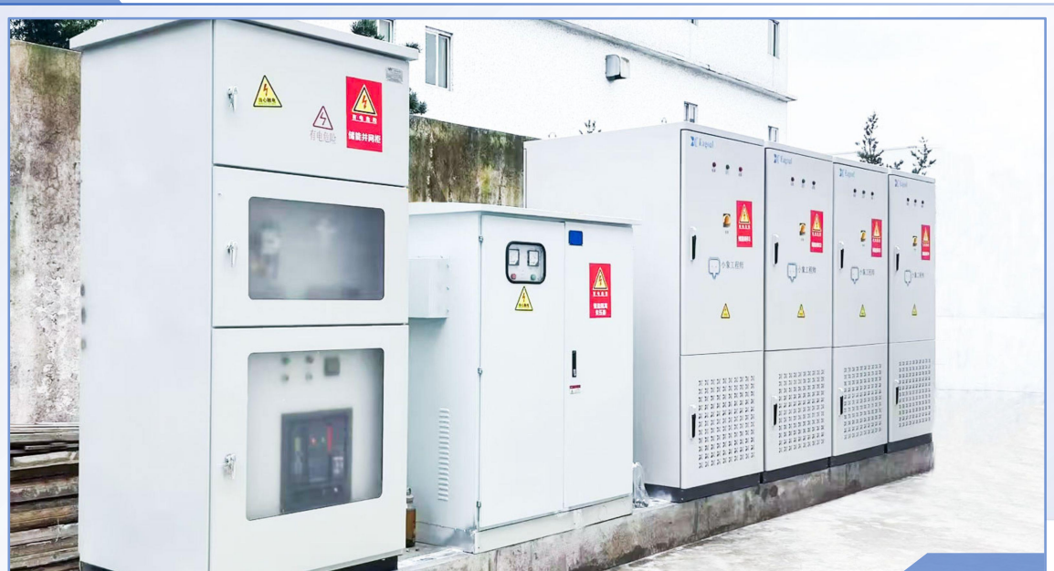
Industrial and commercial energy storage Guangdong Jieyang Industrial and Commercial Energy Storage Project
